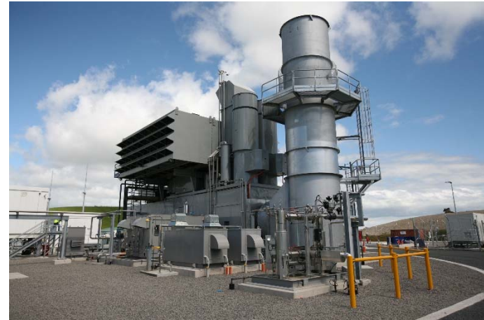
Nova Energy – McKee Power Station
