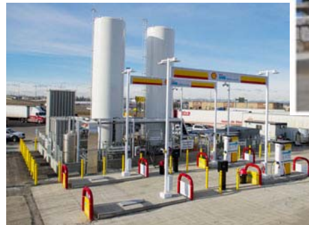
Shell LNG refuelling station - Canada
