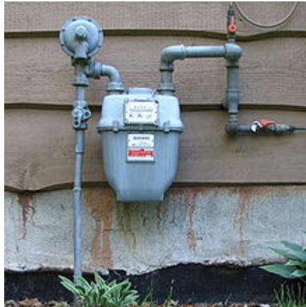
Figure 5 - residential gas meter installation
