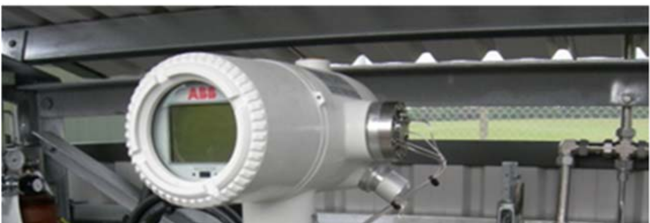
Figure 4: Typical gas analyser (source: Vector Gas Transmission Asset Management Plan 2013)
