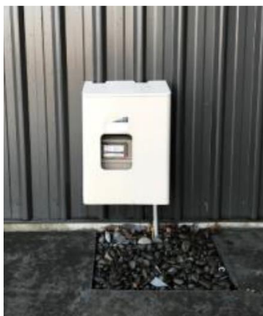
Figure 7 - Residential gas meter installation
