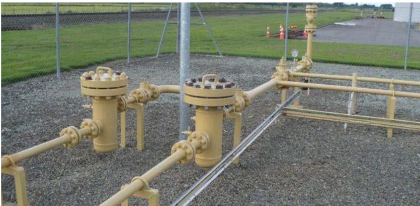
Figure 3 - Filters at the start of two metering 'streams' on a transmission system delivery point
